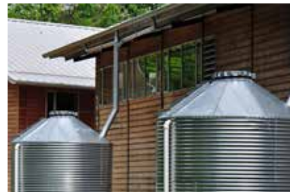
Rainwater Capture and Reuse
