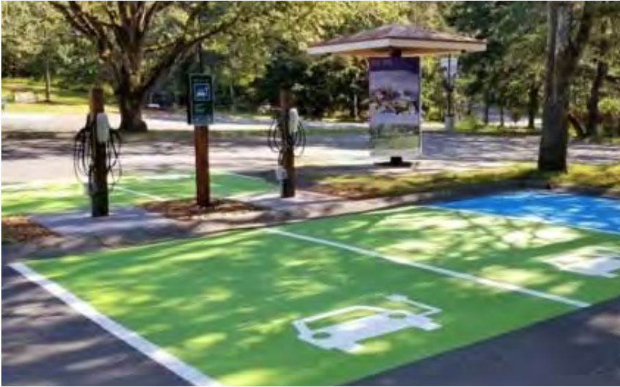
Electric vehicle charging stations
